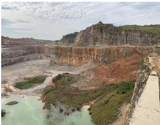
Landslide Hazard Site in Block A of the Steep Slopes of the Xintangpo Mining Pit
